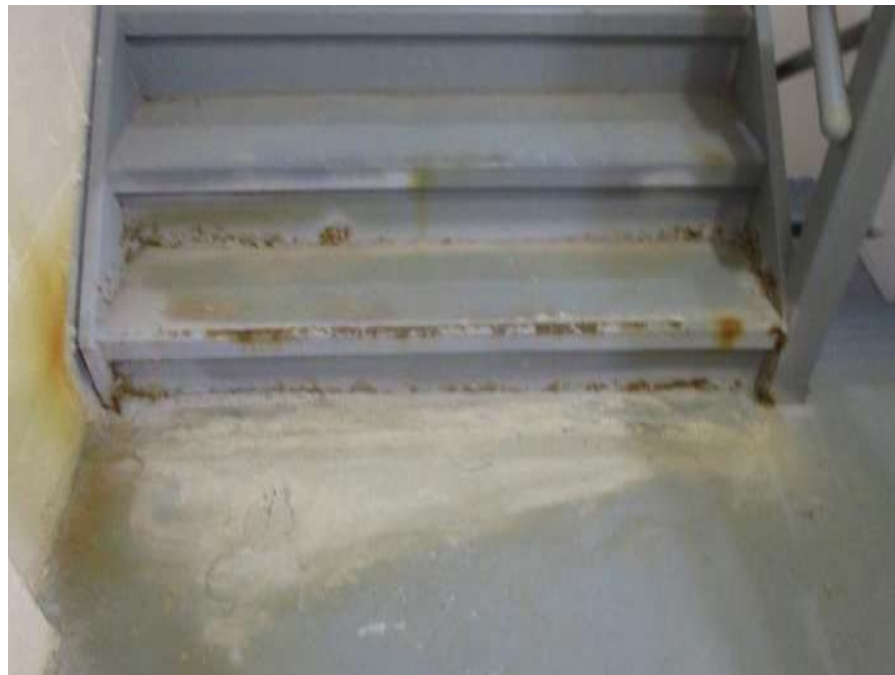
Photo #26 – Typical Corrosion at Stair Treads
