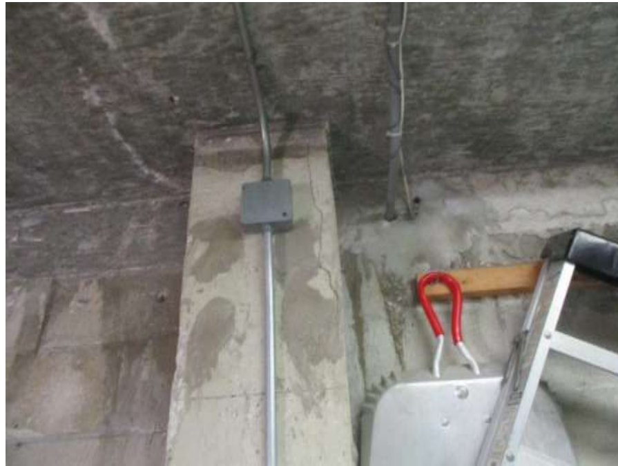
Photo #17 – Isolated Spalling Concrete at Column in Maintenance Room
