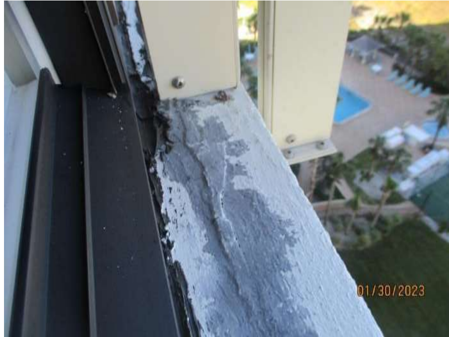
Photo #13 – Damaged Window Sill w/ Previous Repair. Unsealed Fasteners into Sill
