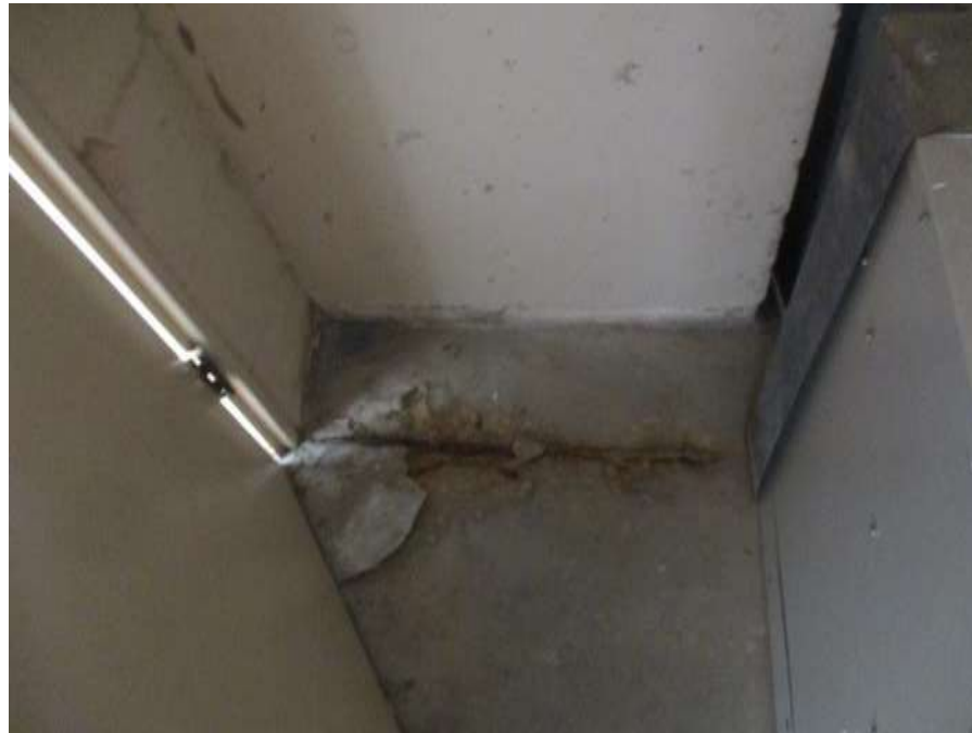
Photo #19 – Typical Spalling Concrete at Utility Closet Threshold
