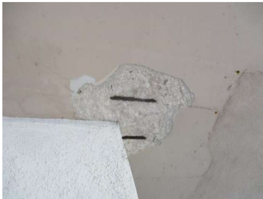
Photo #20 – Spalling Concrete with Exposed Rusty Rebar
