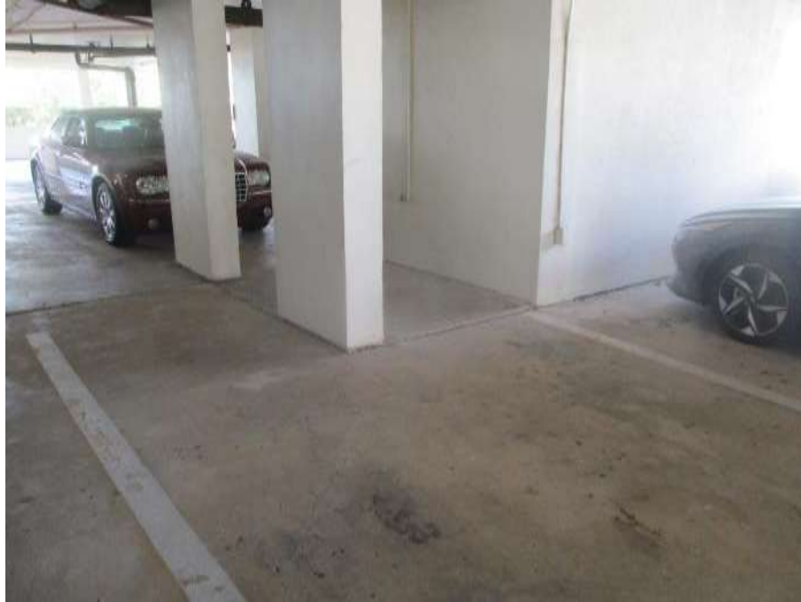
Photo #31 – Settlement of Slab on Grade at Under Building Parking. Potential Trip Hazard due to Raised Portion of Slab at Control Joint
