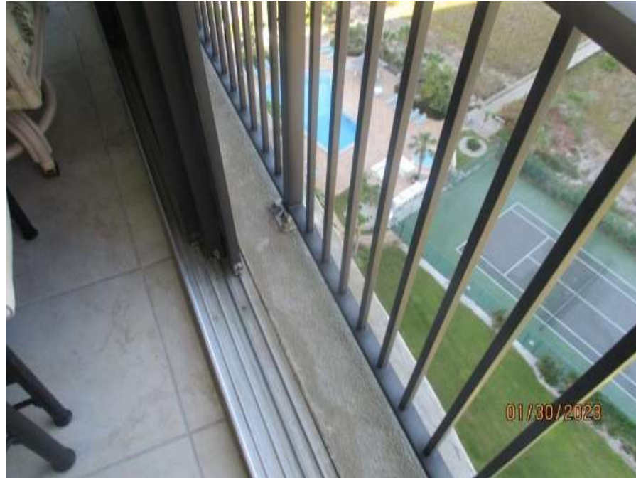
Photo #11 – Typical Balcony with Waterproofing at Slab Edge (Railings Installed Directly to Deck)
