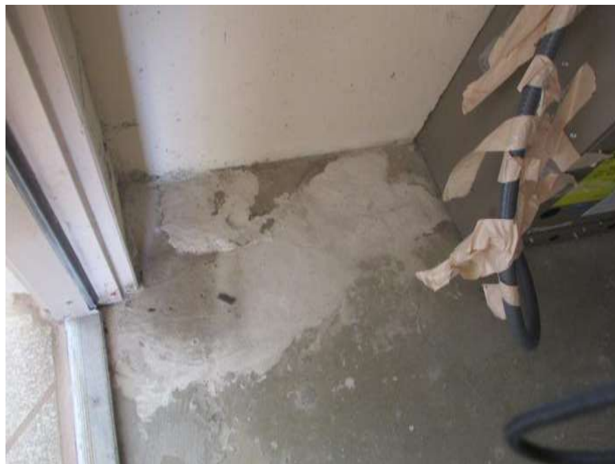
Photo #18 – Typical Spalling Concrete and Failed Previous Repair at Utility Closet
