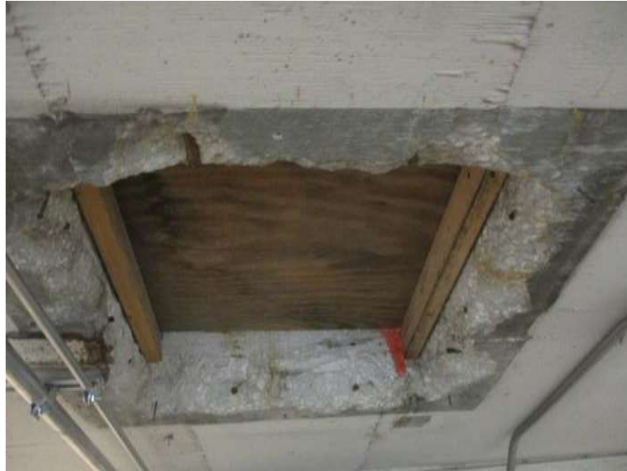
Photo #7 – Roof Access Closed off with Wood Framing with Spalling Concrete and Signs of Water Intrusion
