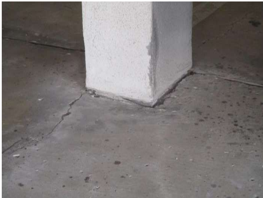
Photo #32 – Evidence of Slab on Grade Settlement at Existing Column. Slab Lower than Column Stucco
