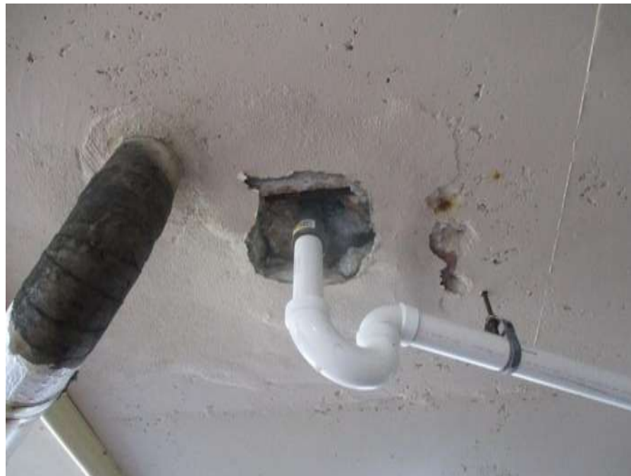
Photo #24 – Isolated Concrete Spalling at Plumbing Penetration Garage Ceiling
