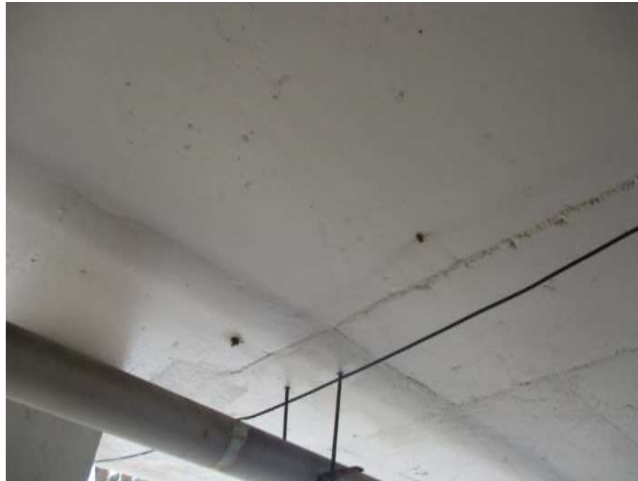
Photo #23 – Abandoned/Broken Pipe Hangers with Corrosion in Garage Ceiling
