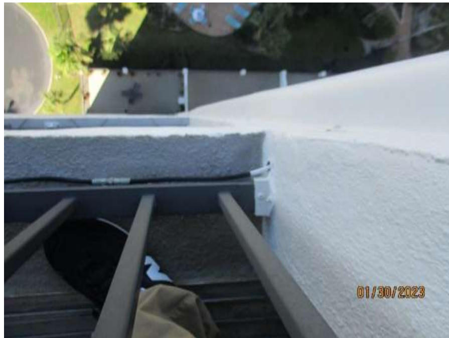
Photo #16 – Typical Unsealed Cable TV Wall Penetration
