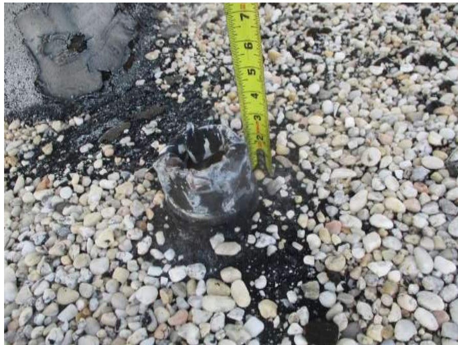
Photo #4 – Height of Roof Vent and Scour Below Code Required 8" Minimum
