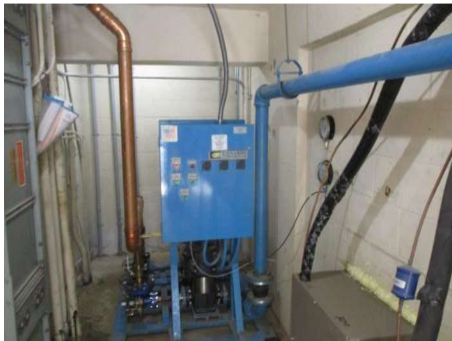
Photo #28 – Domestic Water Equipment Visually in Working Order
