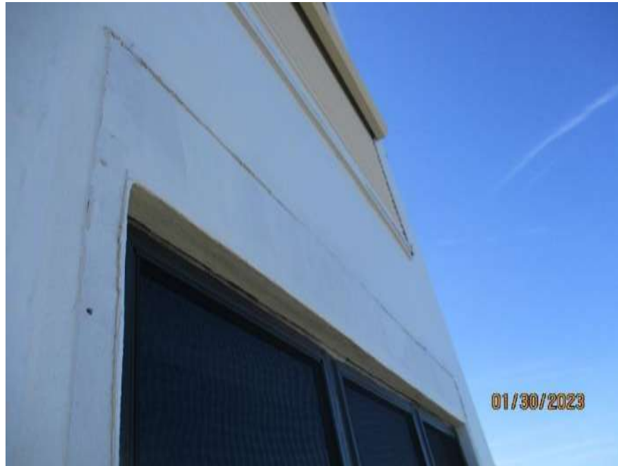
Photo #15 – 1201 West Elevation Window Header Cracked and Delaminated Stucco, Unsealed Fastener Holes from Removed Shutter
