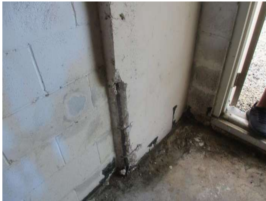
Photo #6 – Spalling Concrete at Storage/Electrical Room at Roof
