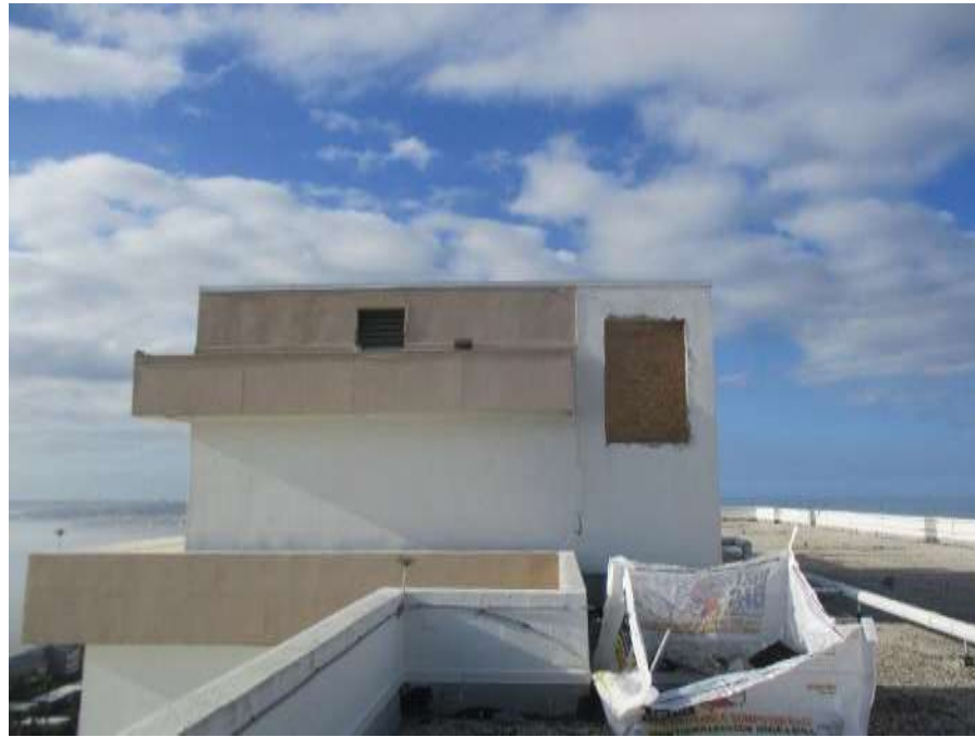
Photo #5 – Elevator Tower Ongoing Elevator Work Wall Opened to Allow Access for Equipment
