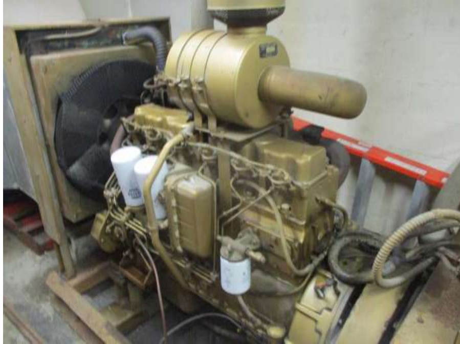
Photo #29 – Emergency Generator Visually in Working Order
