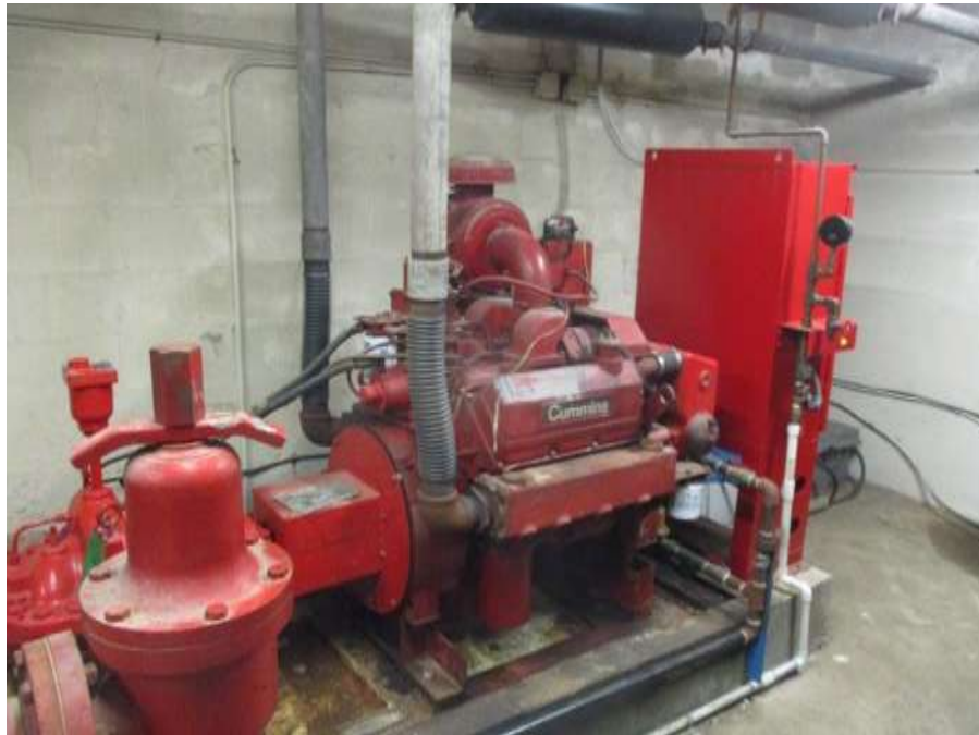
Photo #30 – Fire Pump Visually in Working Order
