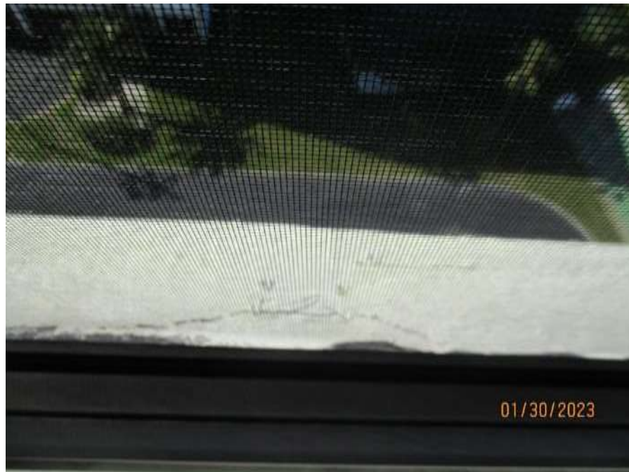
Photo #14 – Typical Cracked Window Sill
