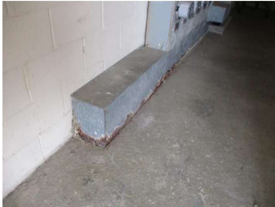
Photo #27 – Typical Corrosion of FPE Meter Panel
