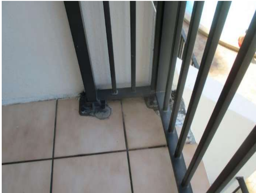
Original Tile Damaged Exposing Slab Edge with No Apparnet Waterproofing Under Tile
