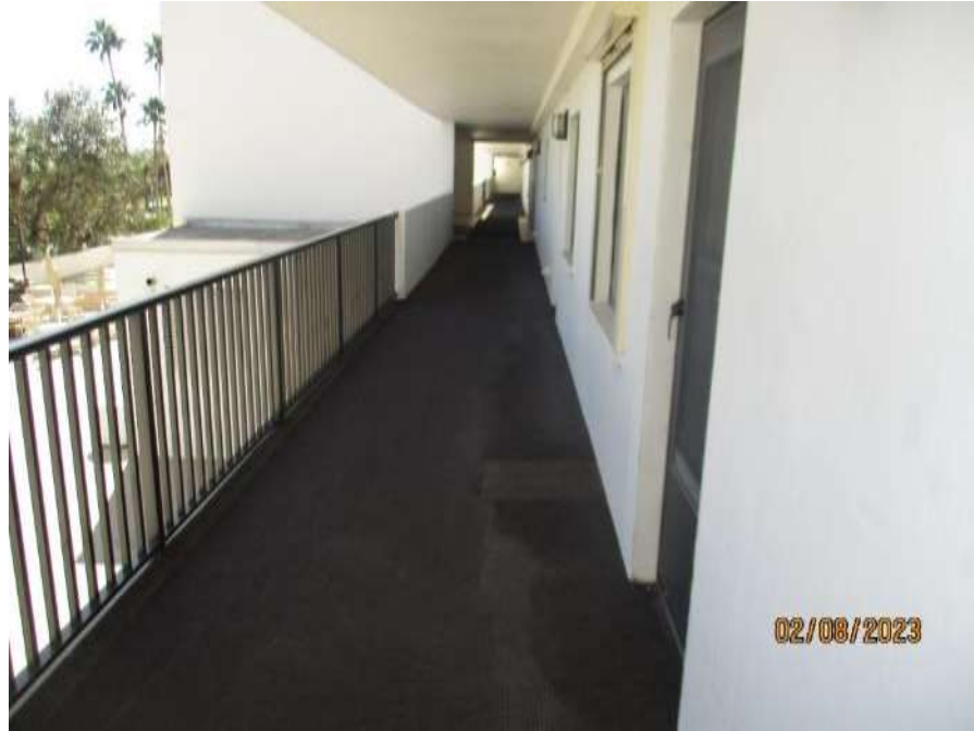
Apparent Water Ponding Staining at 3 rd Level Walkway
