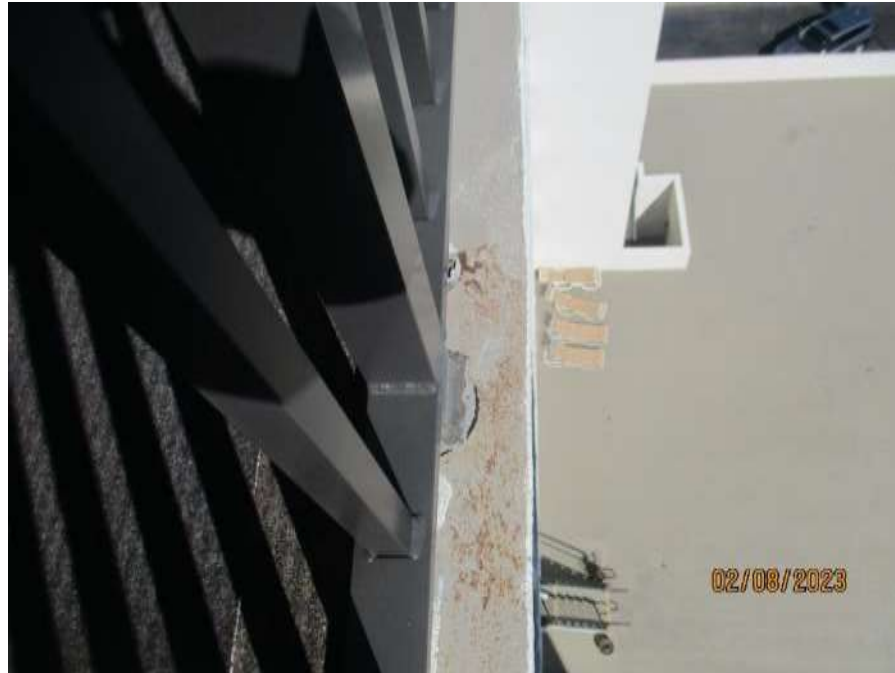
Post Pocket Below Slab Allowing Water to Pond and Damage to Slab Edge Waterproofing
