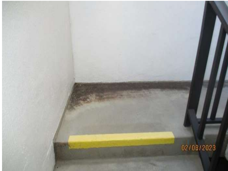
Ponding Staining at Stair Landing
