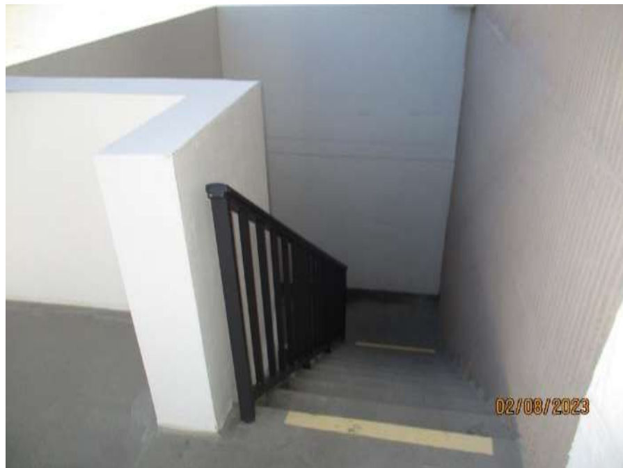
Typical Terrace Deck Stairs to Garage with Non Code Complaint Railings (36" Height 6" Picket Spacing)
