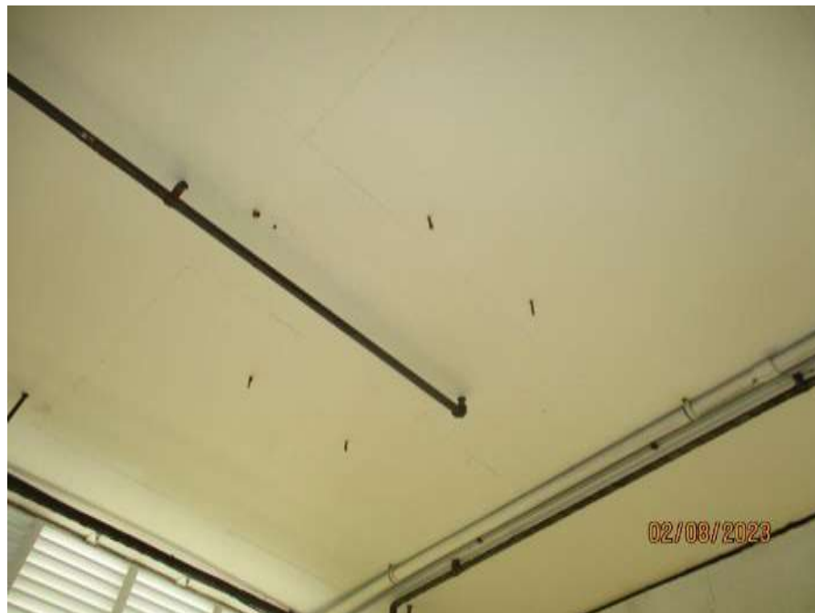
Abandoned Corroded Metal Pipe Hangers Remain in Ceiling
