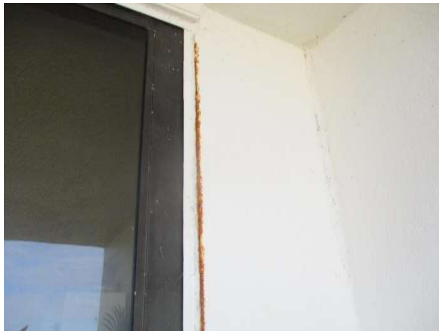
Rusted Corner Bead Stucco Accessory
