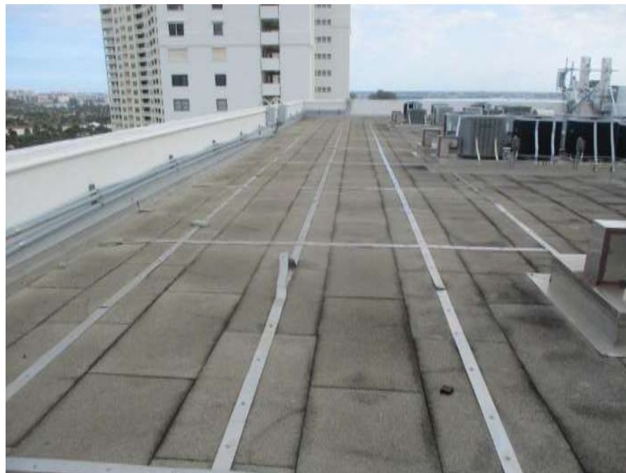
Broken Strapping and Missing Fasteners at Roof System
