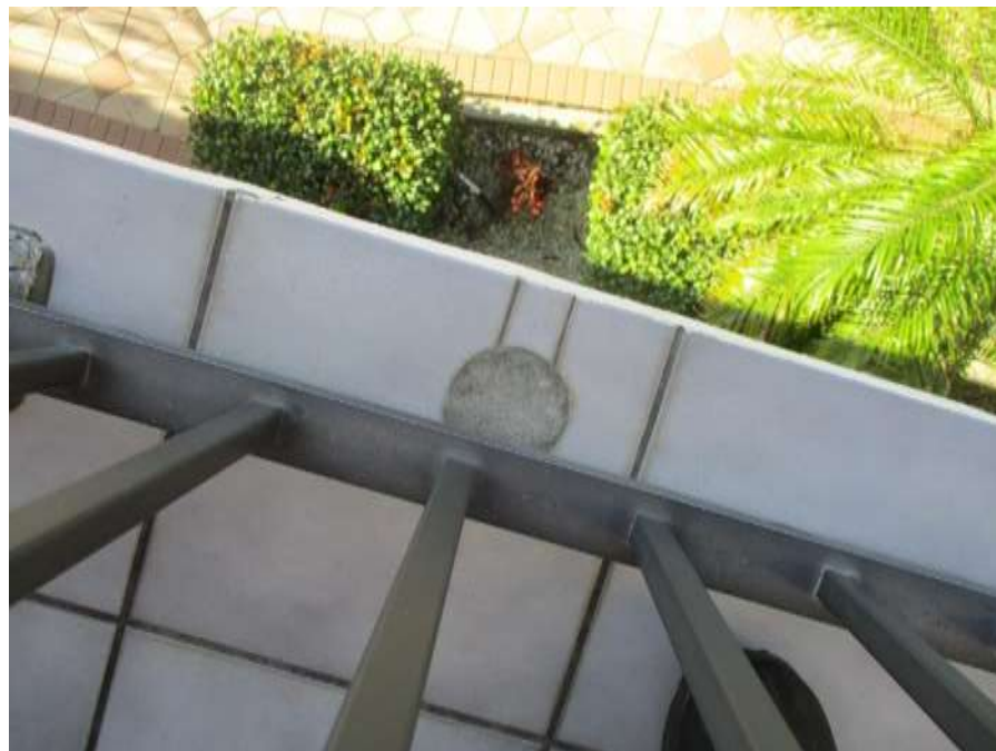
Typical Original Tile at Balcony With Old Post Pocket from Original Railing.
