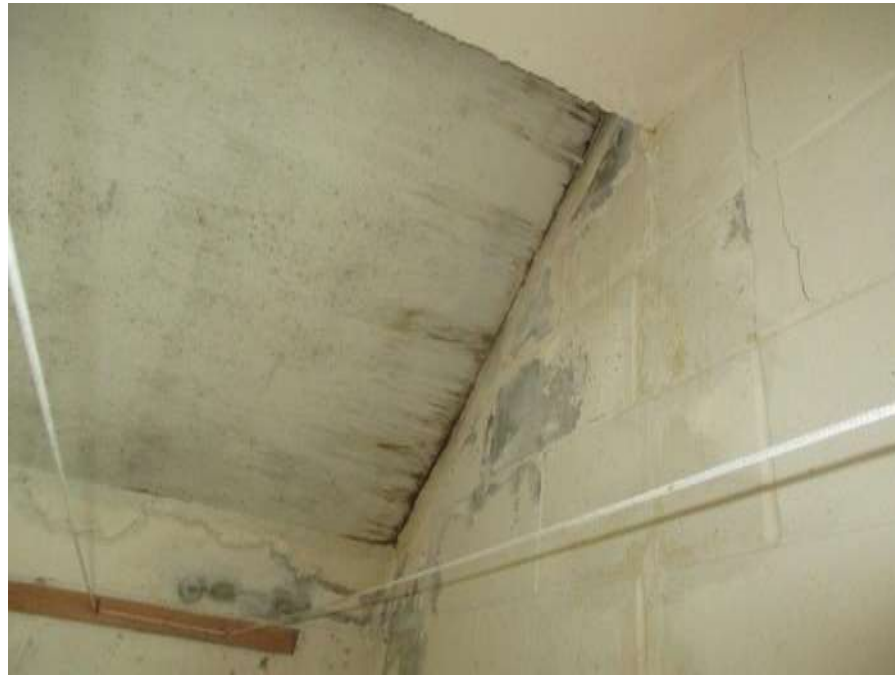
Water Intrusion Indicators into Balcony Closet
