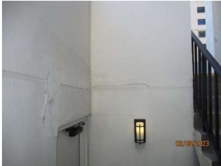
Cracking Stucco and Spalling Concrete at Terrace Deck Stairs (South)
