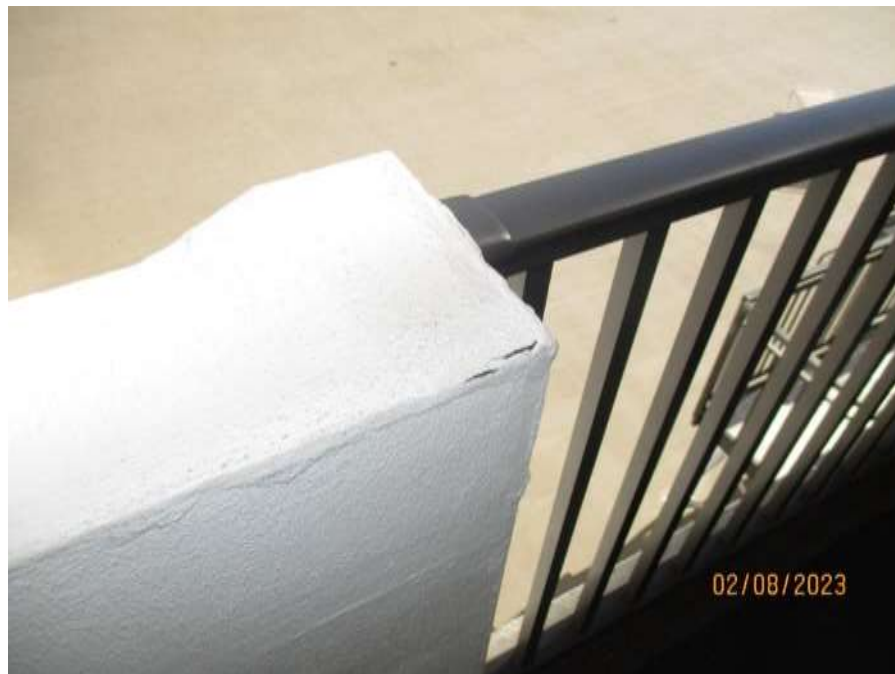
Stucco and Sealant Damage at Guard Wall to Railing Transition
