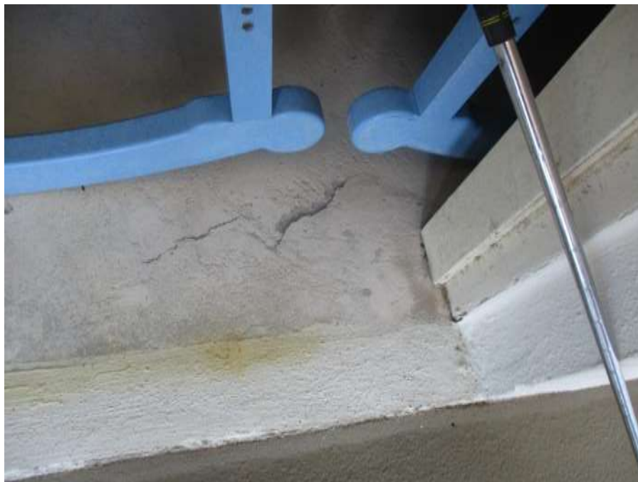
Typical Isolated Concrete Spall in Balcony Closet
